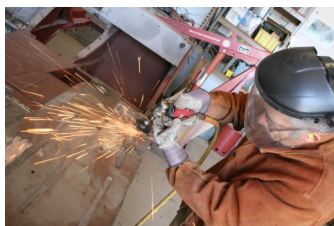
Joe Caetano grinds another rough spot before welding steel plate over rust holes in M151A1 jeep.
